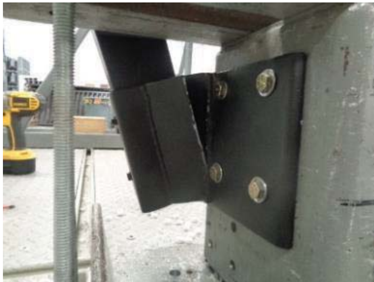
Photo No. 8 Typical Tearing of Outside Corner Bracket
