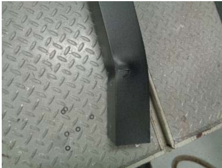
Photo No. 7 Typical Bucking Failure
